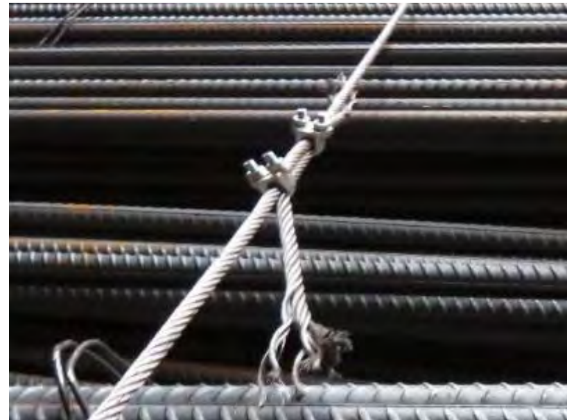
Correct way of using bulldog grips with grips on the live wire. Insufficient number of grips used.
