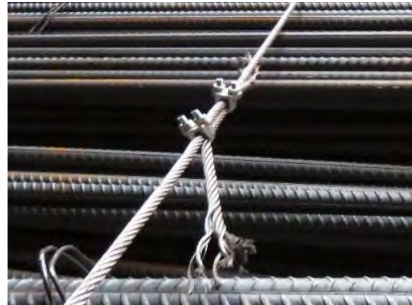
Incorrect way of connecting two wires and using bulldog grips. Insufficient number of grips used.
