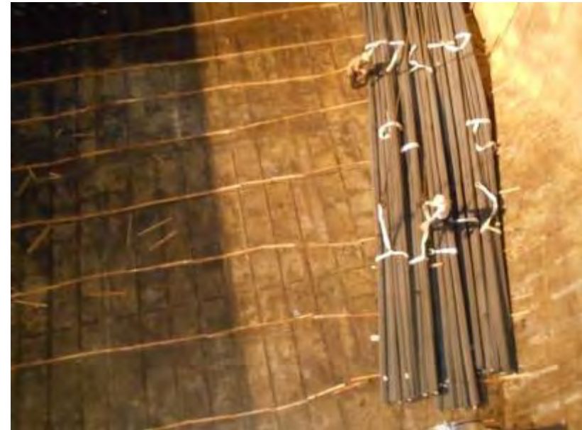
Loading of pre-slung rebars. The spacing of the tank-top dunnage should not exceed 3 meters. In the photograph, the spacing is approximately 2 meters.
