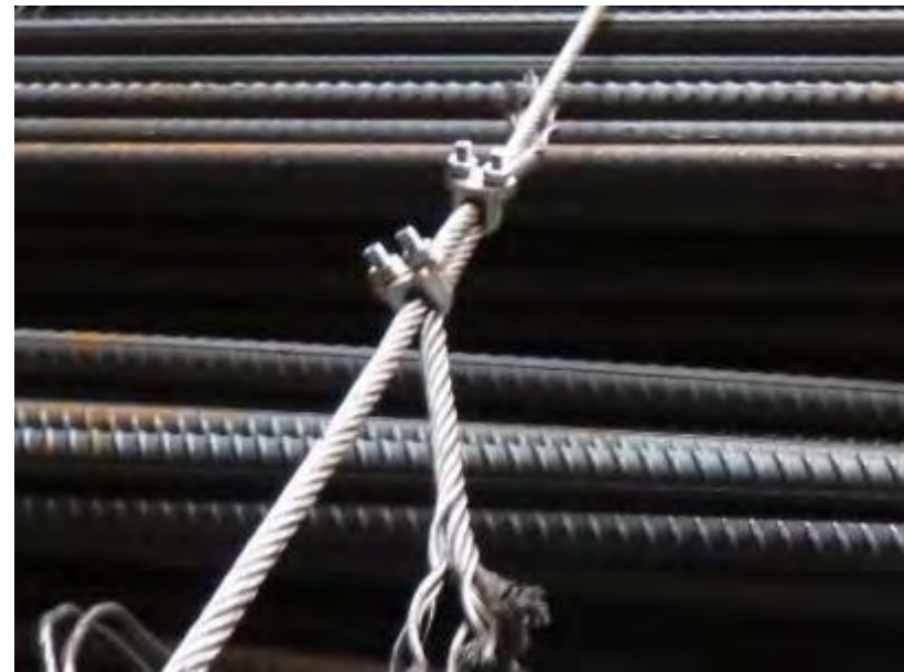
Incorrect way of using bulldog grips with grips on the live wire. Insufficient number of grips used.
