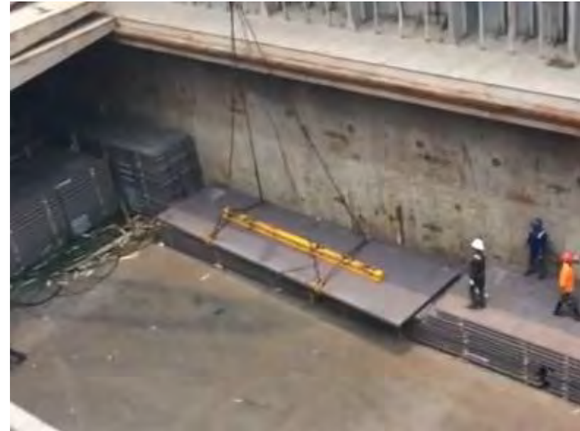
Incorrect handling steel plates under the coaming. The lift is not plumb, and the cargo will sway dangerously towards the center of the hold.
